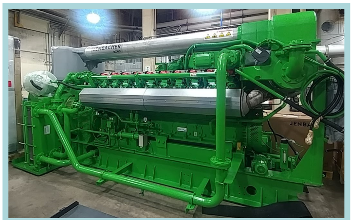
Newly purchased larger capacity, more energy-efficient Jenbacher cogeneration engine.
